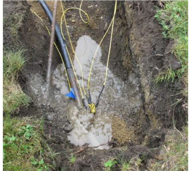
Five tracer wires were used during an HDD pipe installation field test.
