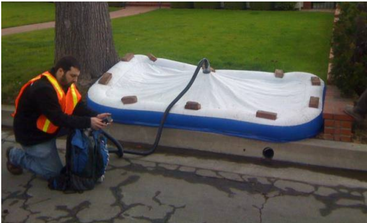
Capturing the gas leak area for rate measurements.
